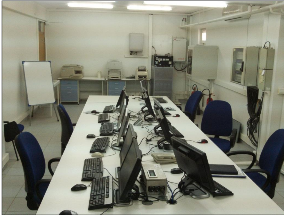
Figure 33: Main center in KOERI
